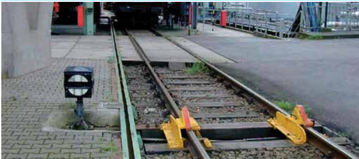
Fig. 6 Derailer at a filling station to prevent other railcars from entering the loading station
