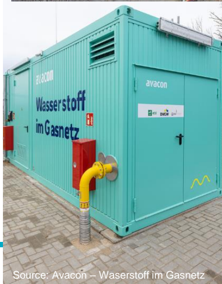
Source: Hydrogen transport in polymer pipes for natural gas distribution – Ten years of experience
